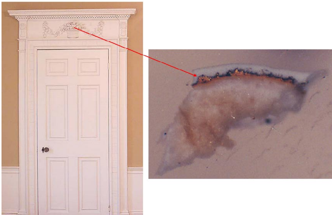
Figure 4. Cross-section revealing gilding beneath white paint in Oak Hill bedroom.
