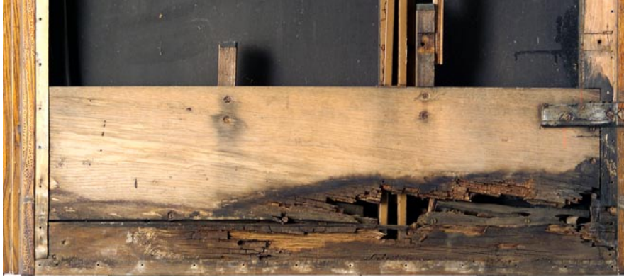
Figure 3. Degraded wood, interior of door.
