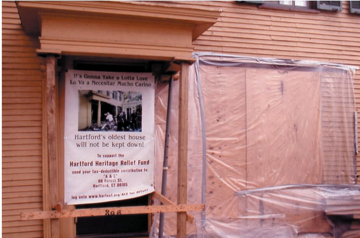
Figure 1. Detail of the exterior, post crash. Note the SUV entry hole to the right of the front door.
