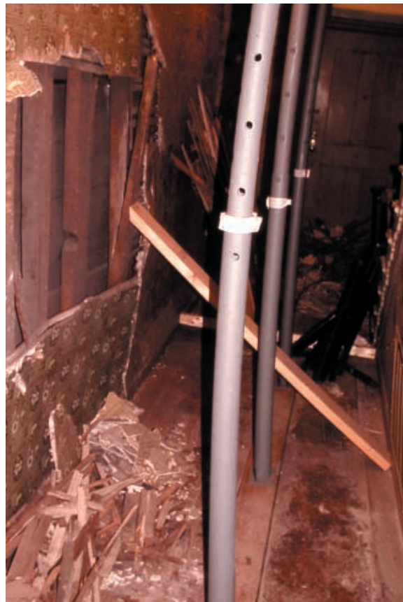
Figure 2. Structural engineers propped up the sagging structure.
