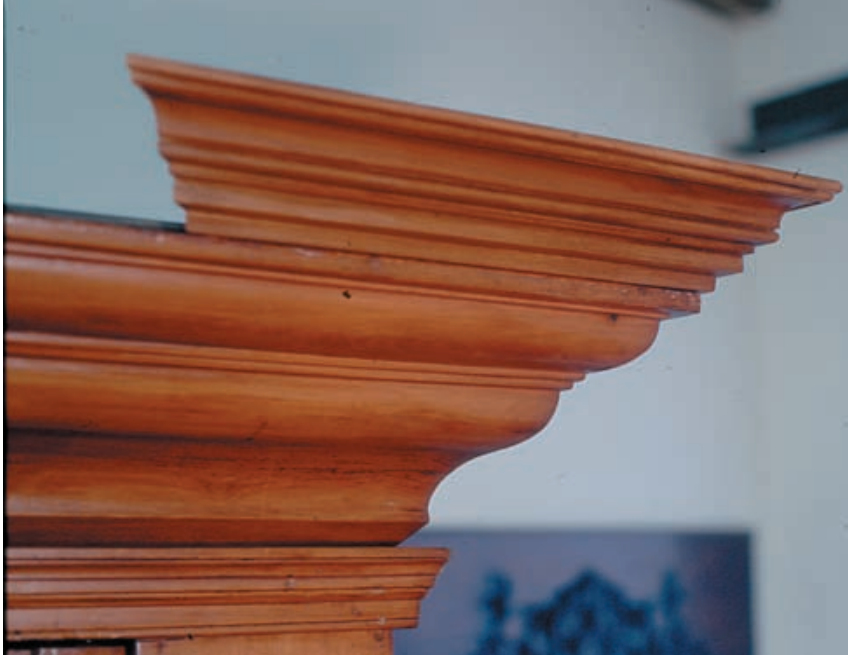
Figure 3. A sample of the proposed restoration was made to show the missing elements.
