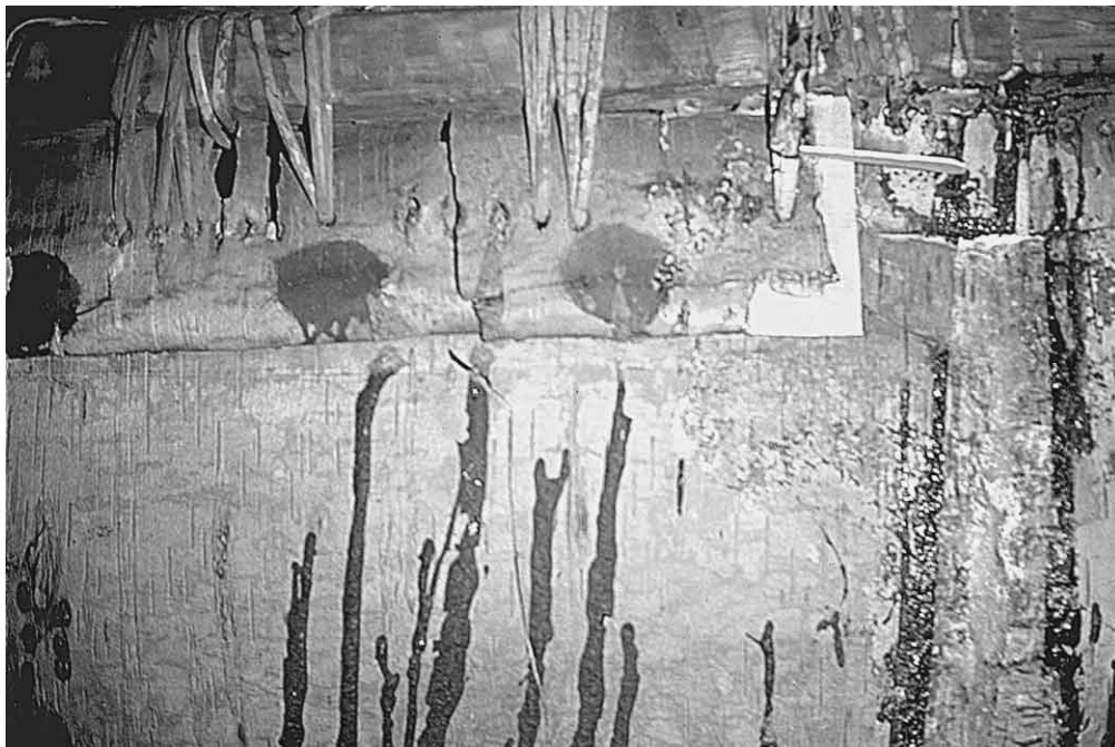
Figure 3: Missing and previously replaced lashings.
